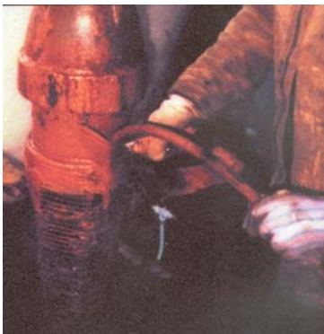
Iron, sulfur, and slime-forming bacteria reduce the effectiveness of conventional well cleaning.
