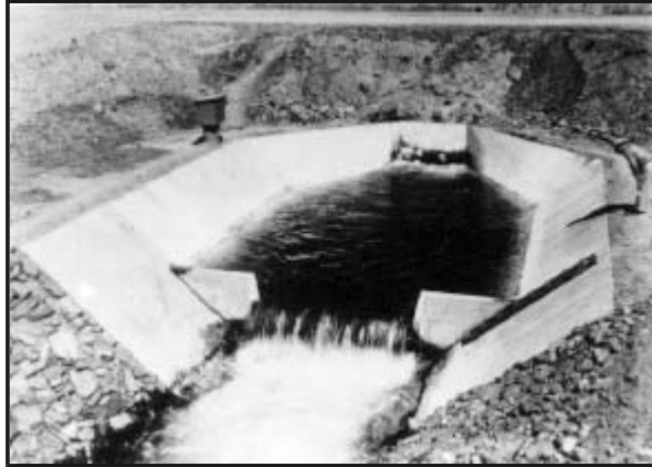
Figure 7-9 -- Cipoletti weir with a well-type head-measuring station.
